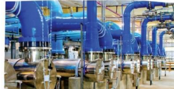
#3 UV LIGHT DISINFECTION AND ADVANCED OXIDATION
