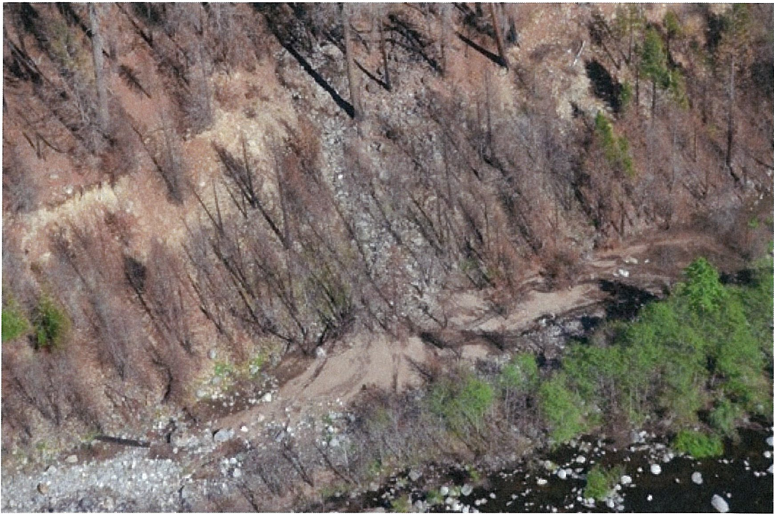
Figure 6: Another example of soil and sediment cascading into Rubicon River, King Fire burn area, April 29, 2015.
